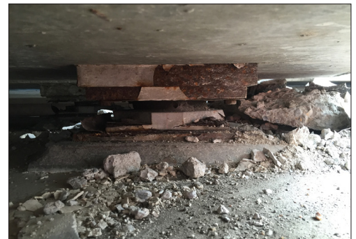
Existing bearing showing excessive corrosion as a result of water leakage from the deck
